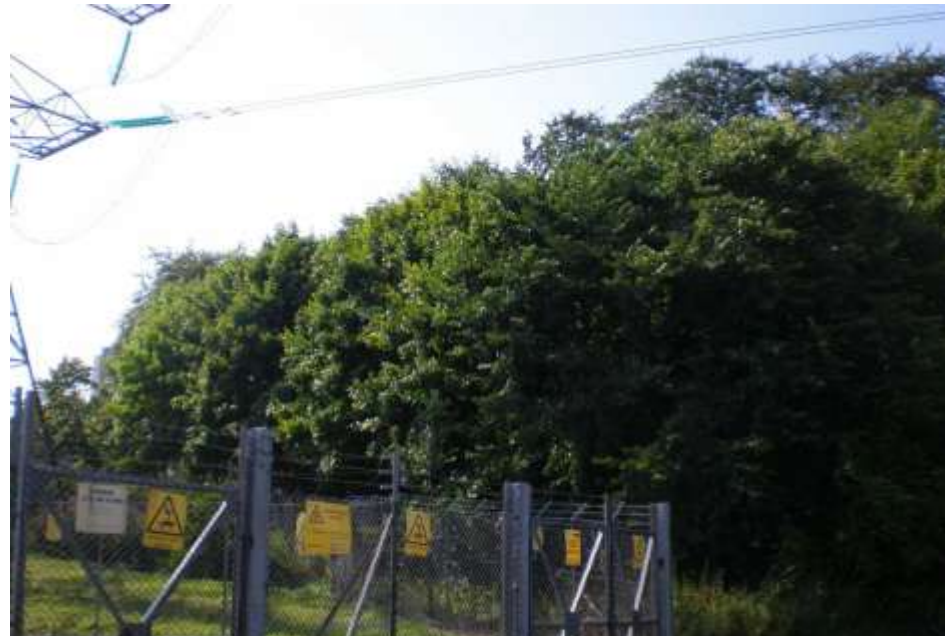
FIG 50: EXISTING SUB STATION COMPOUND
