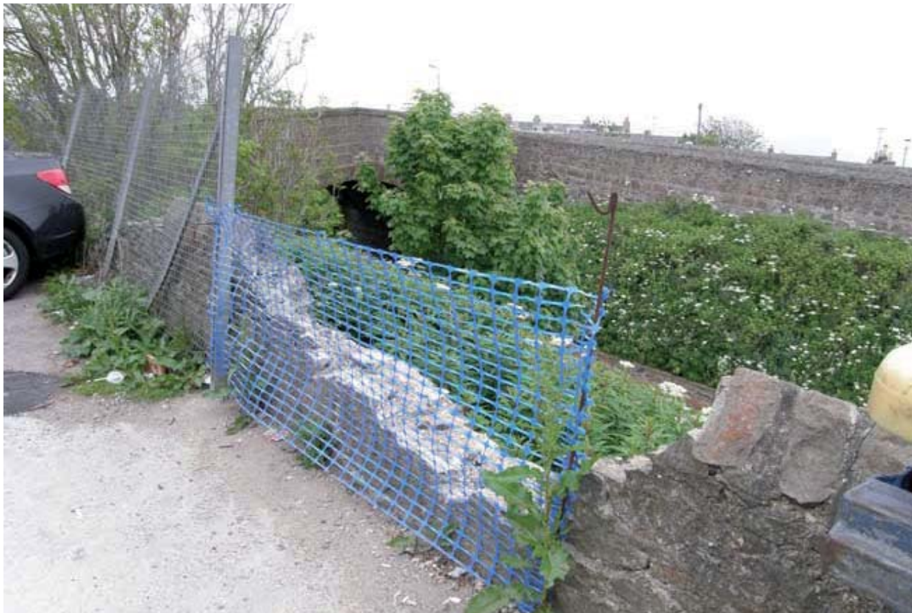
Damaged railway walls
