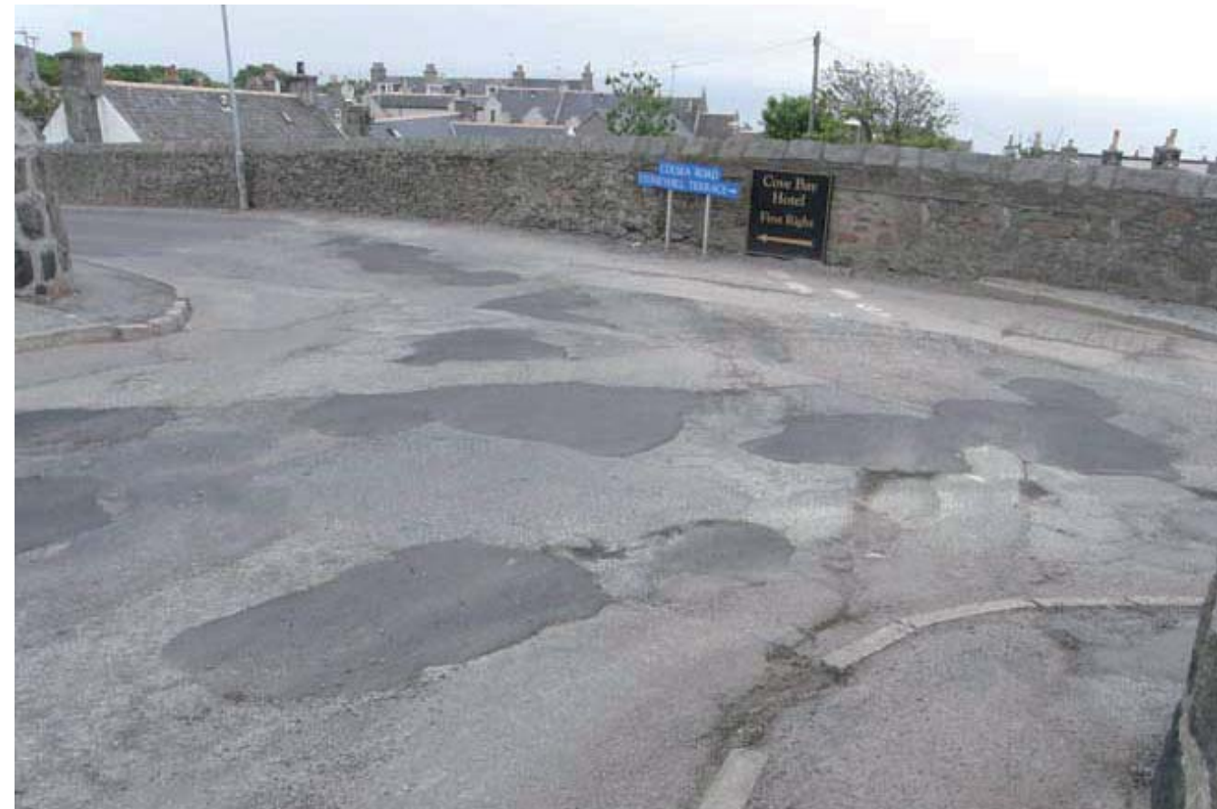
Potholes at railway bridge
