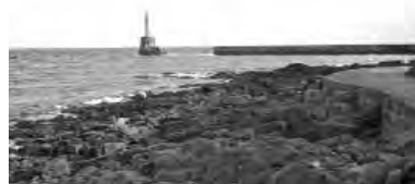
The Breakwater showing damage after the 1937 gale.
