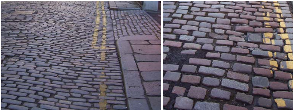
Fig 1: Existing cobbled roads in poor condition
